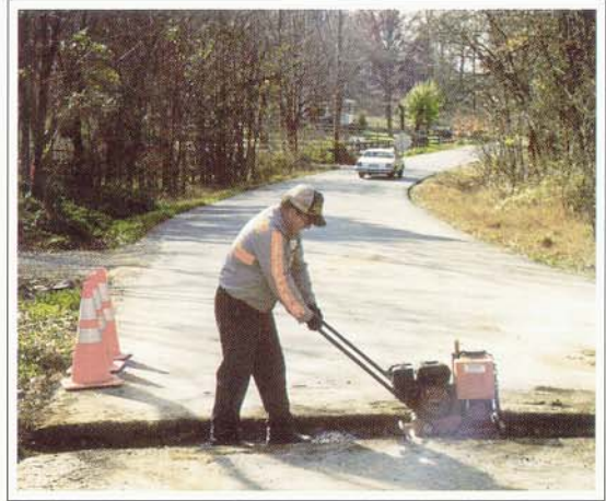
Richard Rollins, Millersville Public Works, uses a plate compactor to pack the subgrade before applying cold patch.
