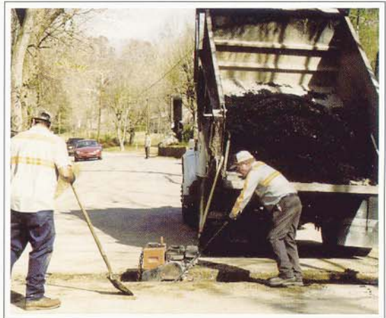
Jerry Schrader, Street Foreman, (left), and Richard Rollins apply EZ Street and pack the hole again with the plate compactor.
