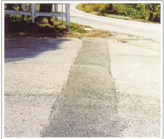
The EZ Street® Cold Asphalt on McMurtry Road in Millersville was completed over six months ago and has had no additional repairs. Thirty percent of the 1200 vehicles that use this road daily are commercial vehicles.
